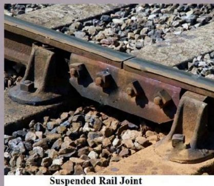
Suspended Rail Joint
