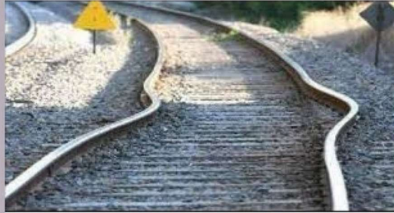
Buckling of Rails
